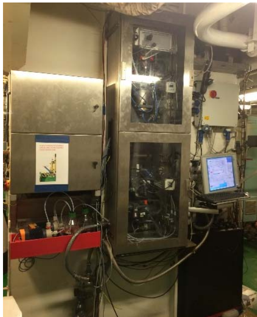
FerryBox in the engine room on CV Hafnia Seaways
