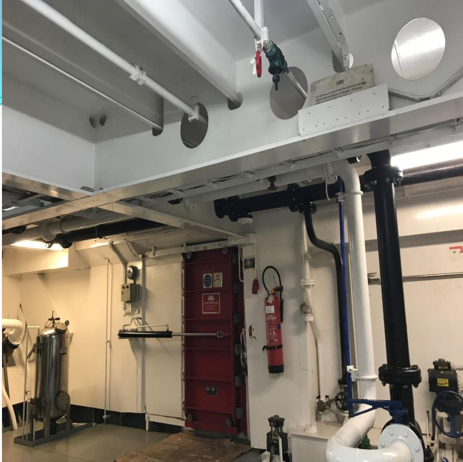
Entrance to the room where the FB will be installed. Photo taken inside the room.
